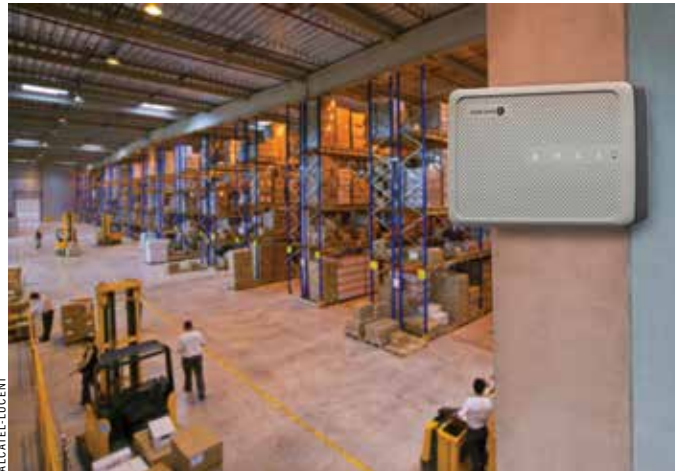
Small cells are used in a variety of interior building settings, from warehouses (pictured here) to grocery stores, to improve cellphone coverage and capacity.
